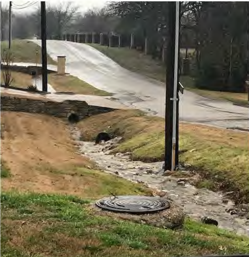
#5 - View of ditch from Santa Fe Circle facing the repair area on Indian Trail
