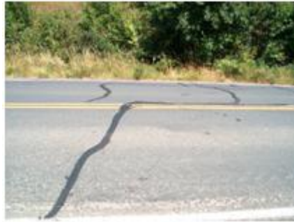
Pavement with crack sealing.
